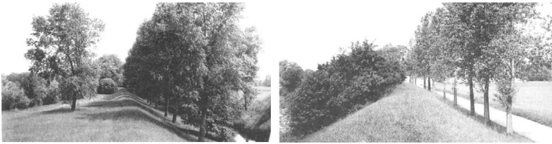
Figure 5: Planted trees and alleys on old levees in Germany (left: flood protection dike at the river Koessnach near with poplars and meadow, 1985 / right: flood protection dike at the river Danube with landside poplar row and waterside bushes and grass/meadow, 1985 / taken from Pflug & Hacker, 1999)
