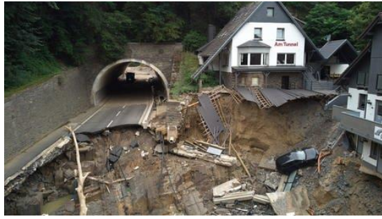
Picture 3: Damages on houses and infrastructure close to the villages Altenahr (Source: www.swr.de )
