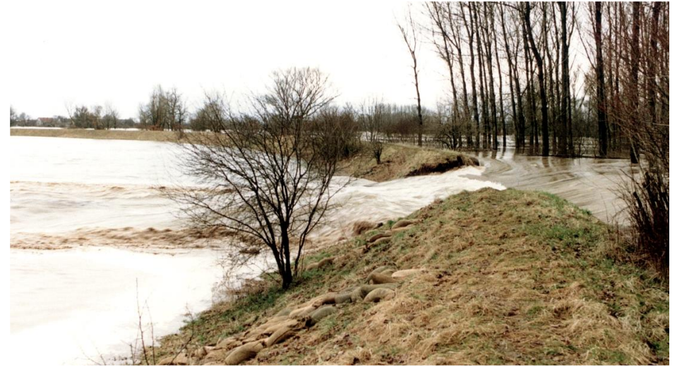
Levee failure at the village Stadldorf during the flood 1988 on the Danube-initial stage (Source: WWA Deggendorf)
