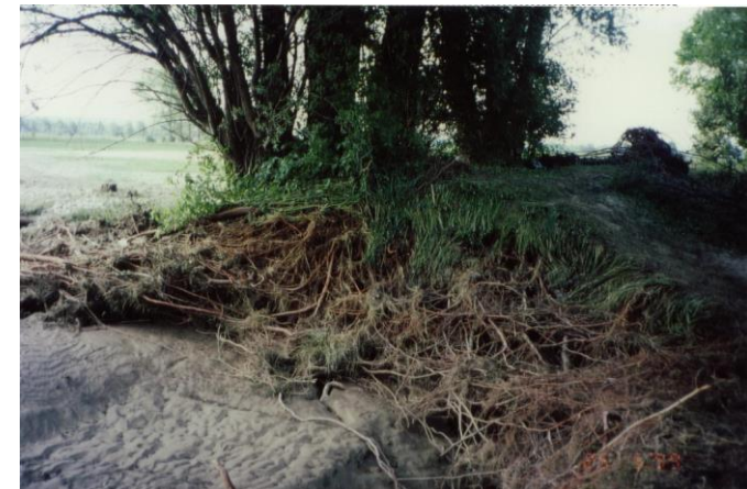
Levee failure on river Ammer after flood 1999 in Bavaria (Source: WWA Weilheim)
