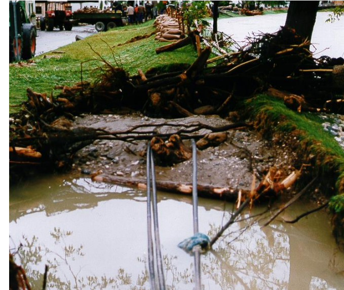
Levee failure on river Loisach (Loisach) after 1999 flood in Bavaria (Source: WWA Weilheim)
