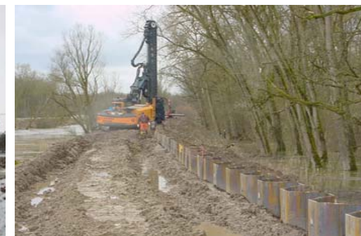
Sheet pile wall in dike at River Danube (Source: WWA Ingolstadt) No. 11
