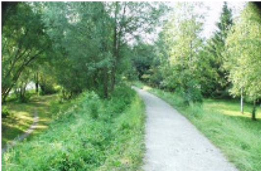
Flood protection dike at the river Mangfall before remediation (Source: WWA Rosenheim)
