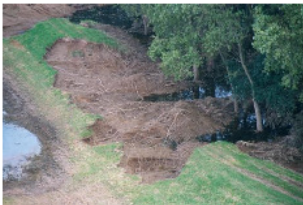
Dike breach during flood incident 1999 at the river Ammer (Source: WWA Weilheim)
