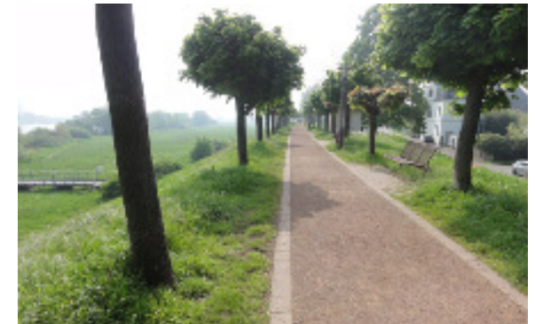
Flood protection dike at the river Rhine, Orsoy, wooded dike (Source: BCE, 2019)
