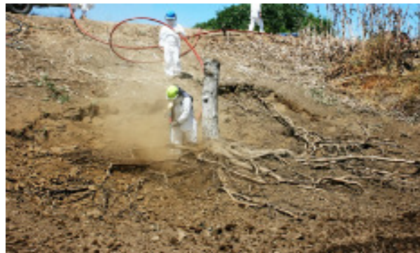
Rooting through embankment Vernalis, California, USA (Source: Berry and Chung, 2013)
