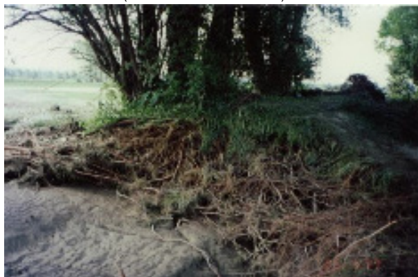
Failed Dike at River Mulde (2002) (Source: Landestalsperren-verwaltung Sachsen)
