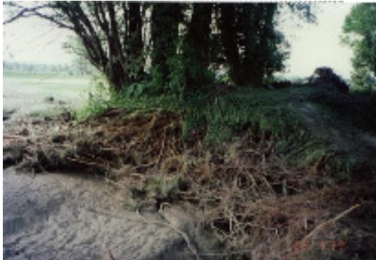
Dyke breach during flood incident 1999 at the river Ammer (Source: WWA Weilheim)
