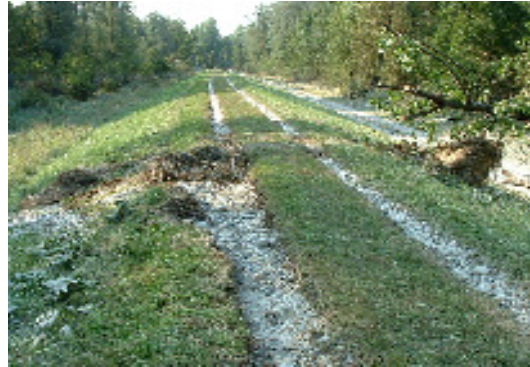
Erosion damages at dyke crest after windthrow lead to overtopping during flood incident 2002 at river Salzach (Source: LfW)
