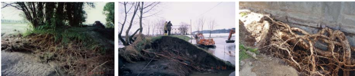
Figure 9. Rooted levees at the River Ammer (left) (Source: WWA Weilheim) and River Danube (middle) (Source: LfW BY) and excavated roots of a poplar at a flood protection wall in Düsseldorf (right)
