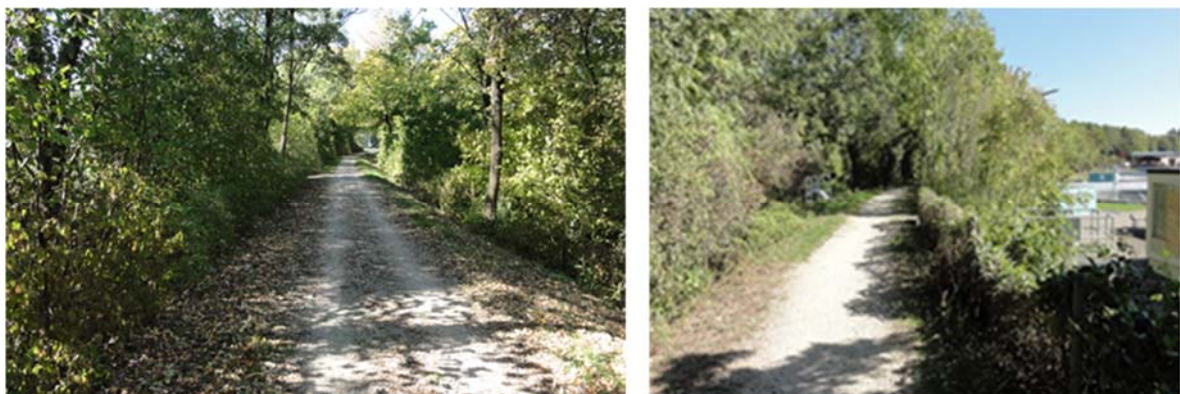
Figure 13. Existing levees along the Neckar River at the city of Nuertingen with large trees on both slopes (taken from Kerres & Haselsteiner, 2018).
