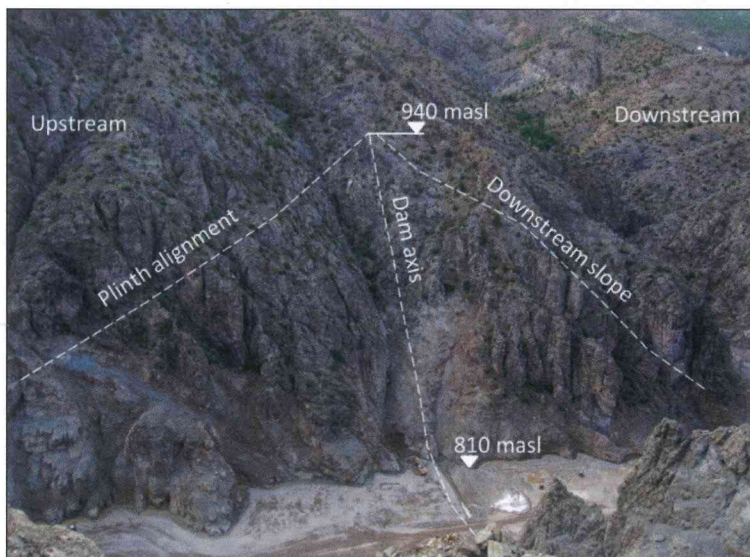
Fig. 2. Left abutment of Arkun main dam site during the initial phase of dam body fill works.
